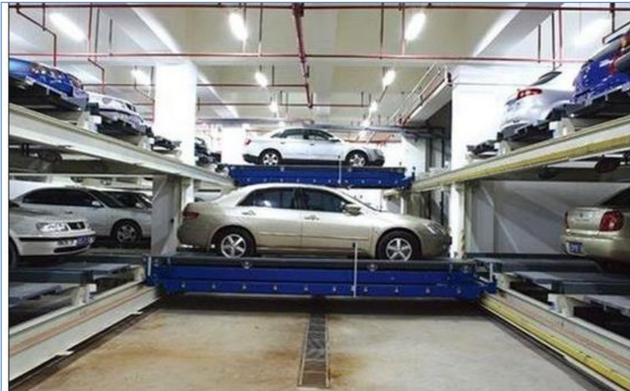
Figure 34 -Improved economies of scale and efficient use of space may be achieved by provision of centralised car parking stations, where provision of onsite car parking is not practical or feasible to achieve.
